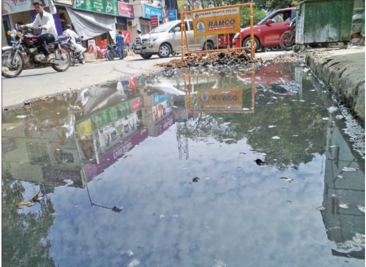
By Our Staff Reporter Sewage water has been overflowing from the manhole chamber at the junction of Thambaiyah Road Extension and Ganapathi Street, West Mambalam for more than 20 days.
